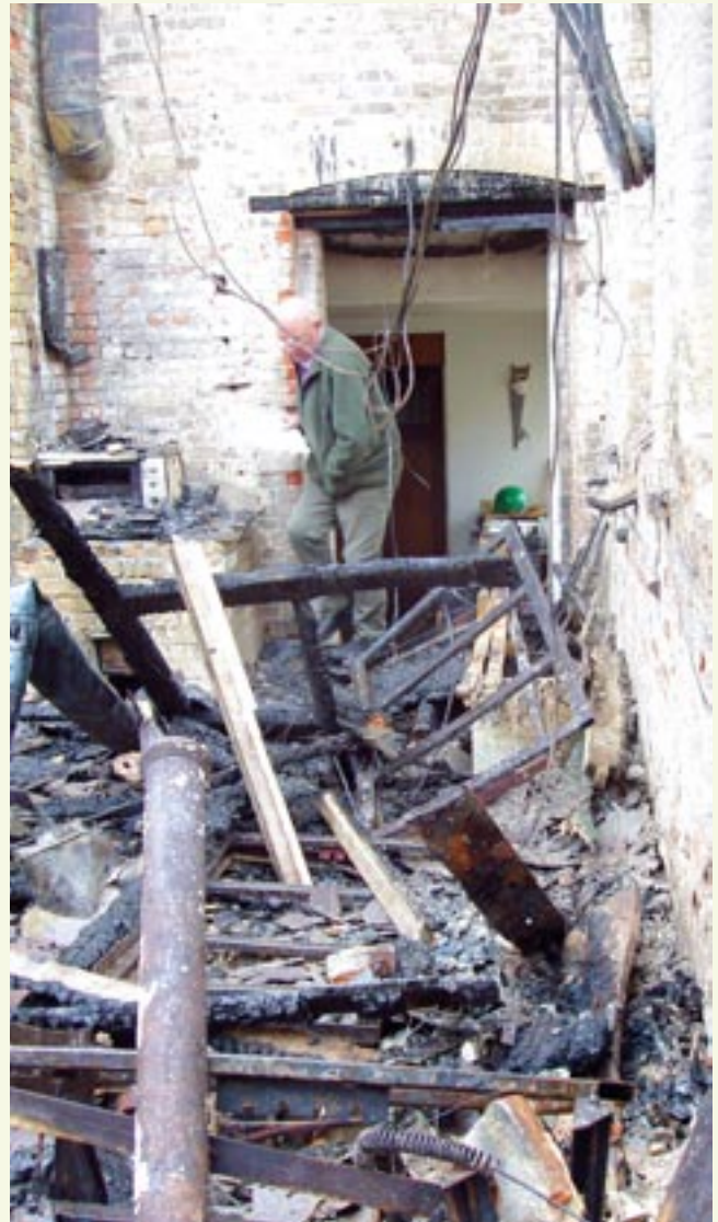
ABOVE: Maurice Bray assesses the damaged at the fire-ravaged Windowcraft Department.
